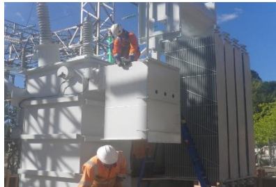
Installed in final location in switchyard
