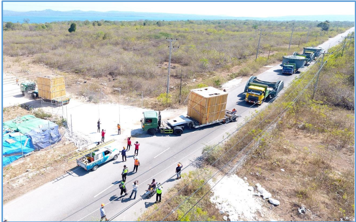
Figure 2 The furnaces arriving on site after transportation from the nearby Tenau Port, Kupang
