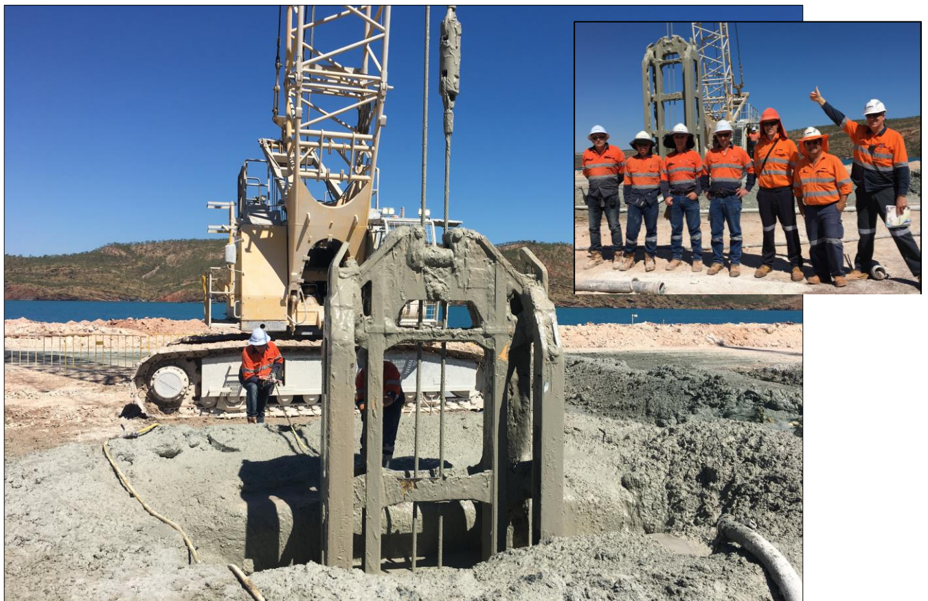
Figure 3: Excavation of final seepage barrier panel - July 2018. Inset: MGX and Keller personnel celebrate completion of the final panel.
