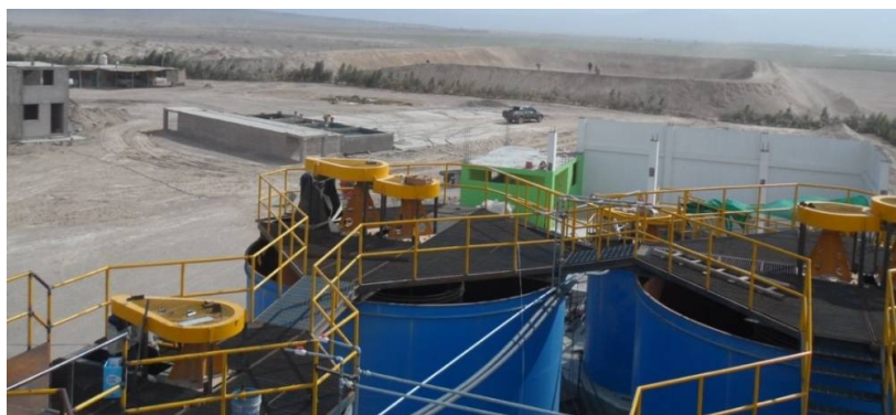
Figure 5: Vista Carbon & Leaching Tanks, with Tailings Dam in the distance.
