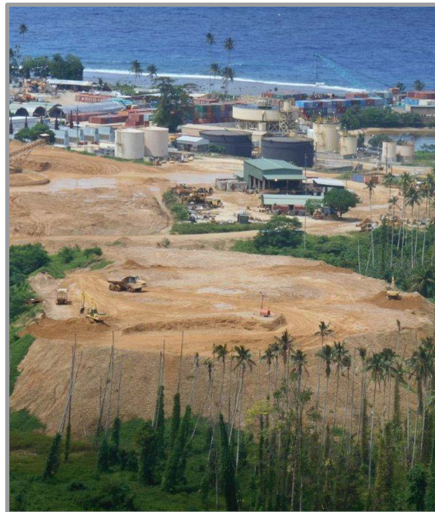
Simberi Operation showing processing plant stockpile, February 2018, photo Liken Paulias
