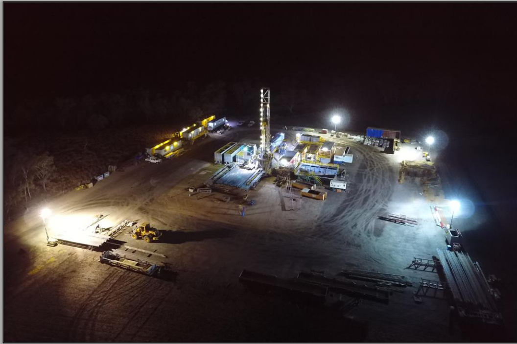
Ensign drilling rig 964 on location of the Armour Energy Myall Creek 4A well.
