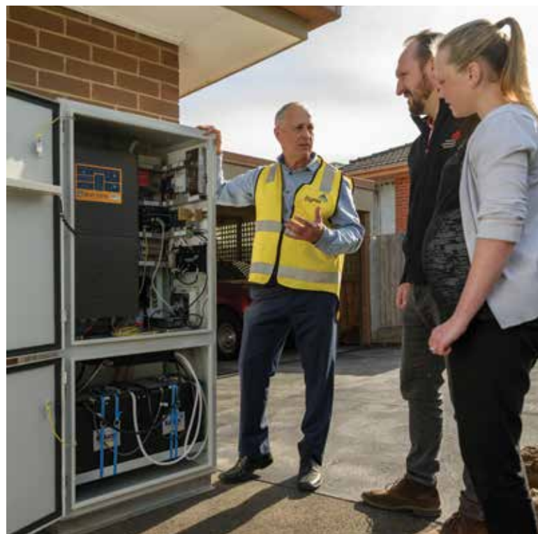
Peter Maruff shows Mooroolbark customers Jeff and Corrine Ward their new residential battery installation.
