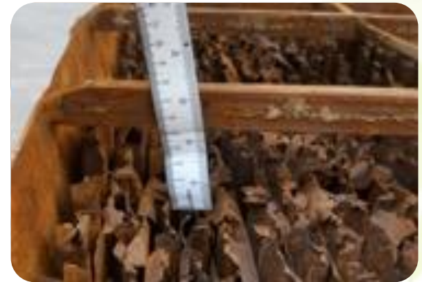
Corrosion of air heater baskets caused by bromine
